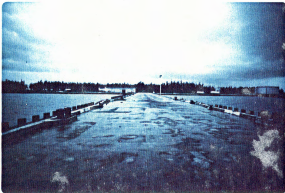
Plate 22. Midway Harbor, view from end of concrete pier looking toward Sand Island
