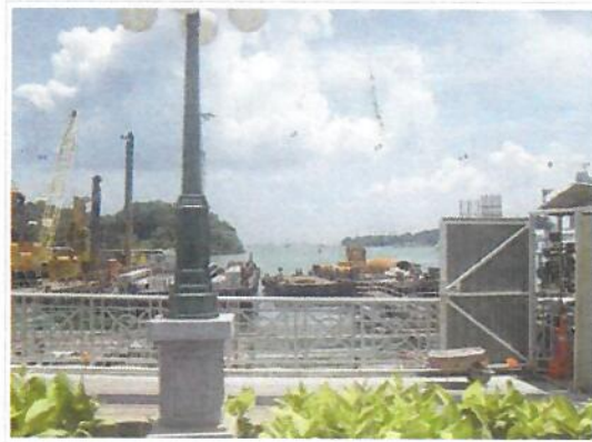
Just before boarding the ferry, a look at the reclamation and dredging going on for the massive Pasir Panjang Container Terminal reclamation project.
