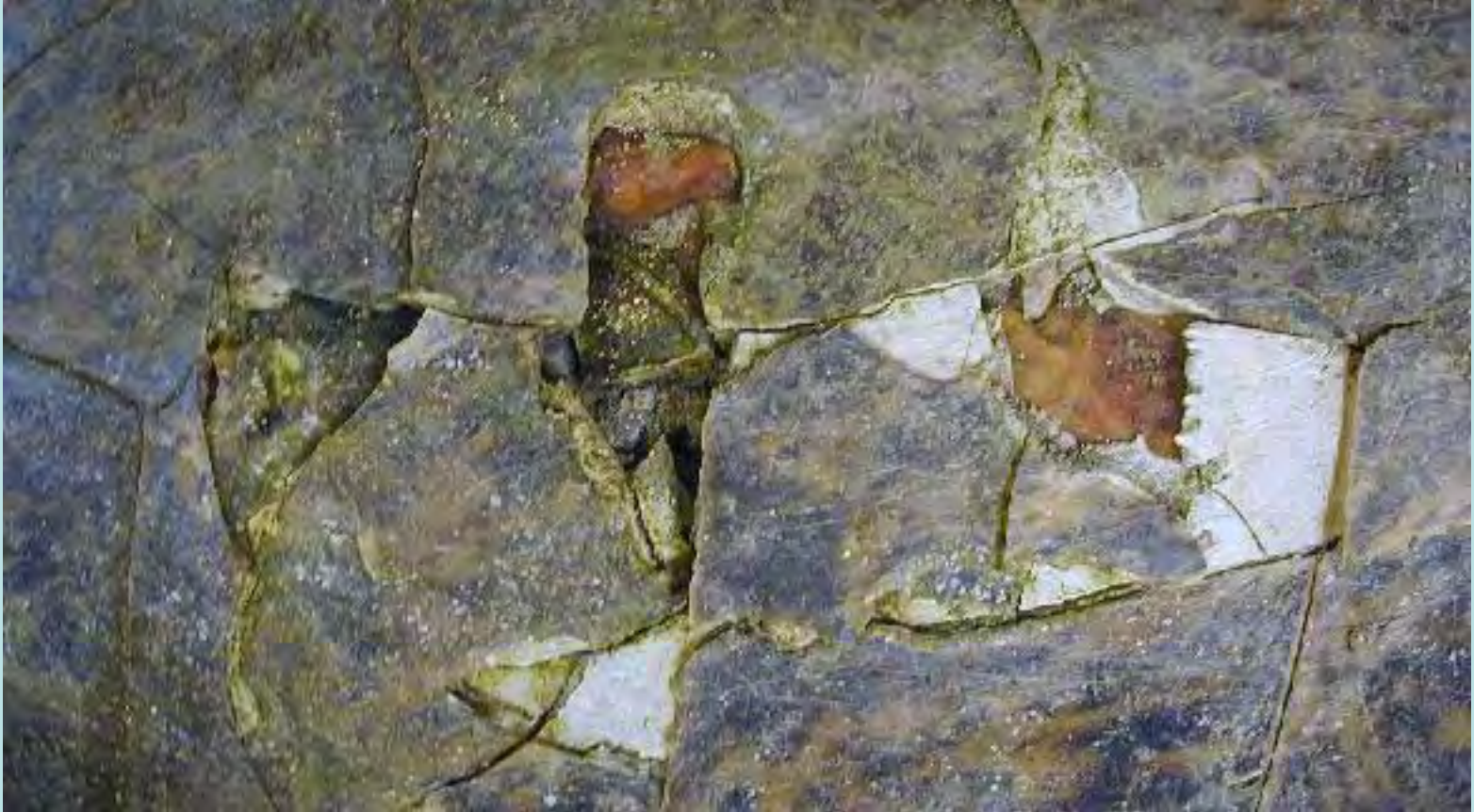
CLOSE UP OF SHELL DAMAGE
