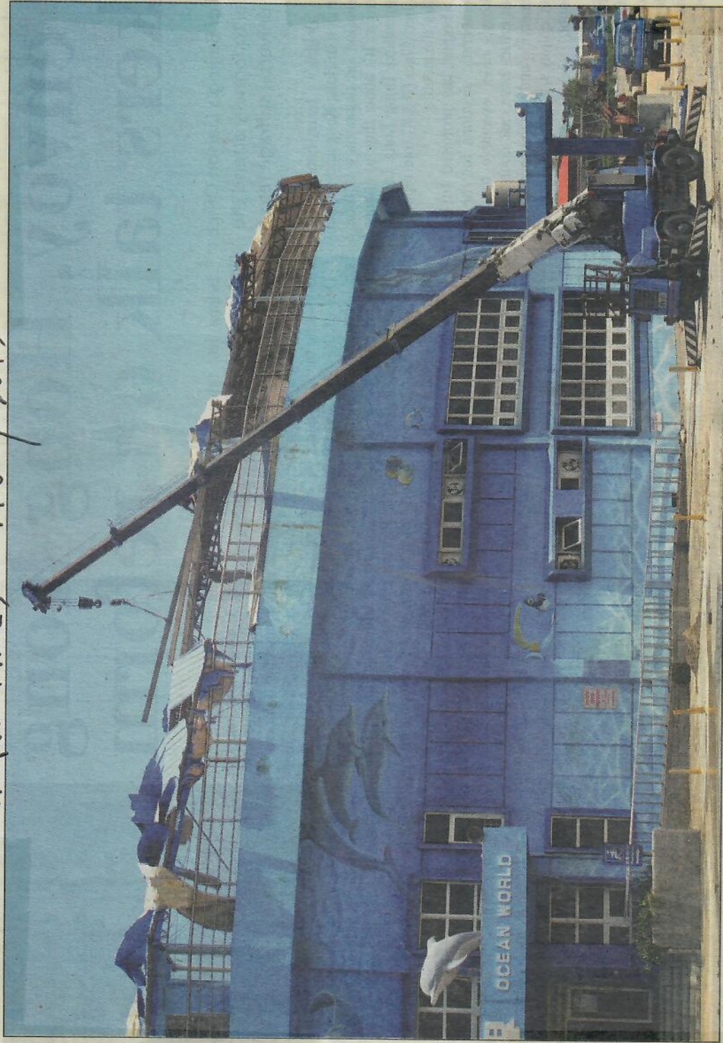
Workers use a crane to dismantle the roof of Yehliu Ocean World in New Taipei City on Sunday after the building was badly damaged by wind and waves during Typhoon Soulik on Saturday.
