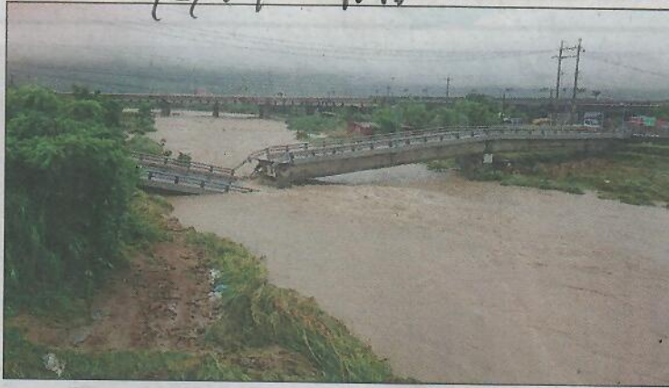
The Huangxi Bridge, which connected New Taipei City's San Jie Tan area with Jinshan Old Street, is pictured after being broken in half by flooding yesterday. PHOTO: COURTESY OF A READER
