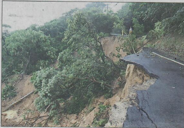
An industrial road connecting Keelung's Zhongshan and Anle districts is pictured after it collapsed due to torrential rainfall. PHOTO COURTESY OF KEELUNG'S ZHONGSHAN DISTRICT OFFICE
