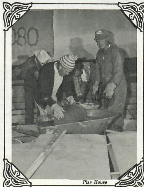
Pouring concrete for seats in new cultural center. L.-R. - Charlie McManon, Vern Krause, Bob Allred, Dickm Davis.
