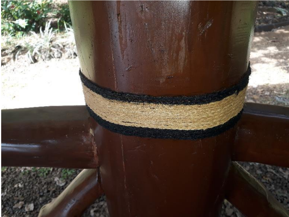
Details of lashings in fale using traditional sinnet (afa) Some lashing work still to be done
