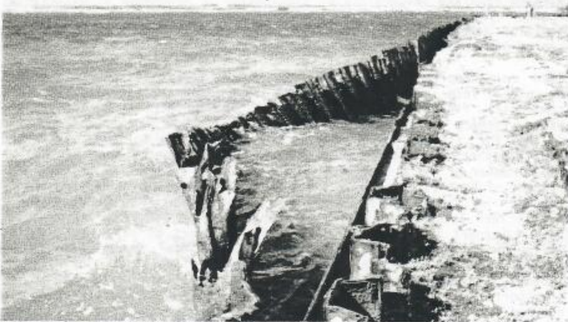
Deteriorated sea wall at Tern Island.
