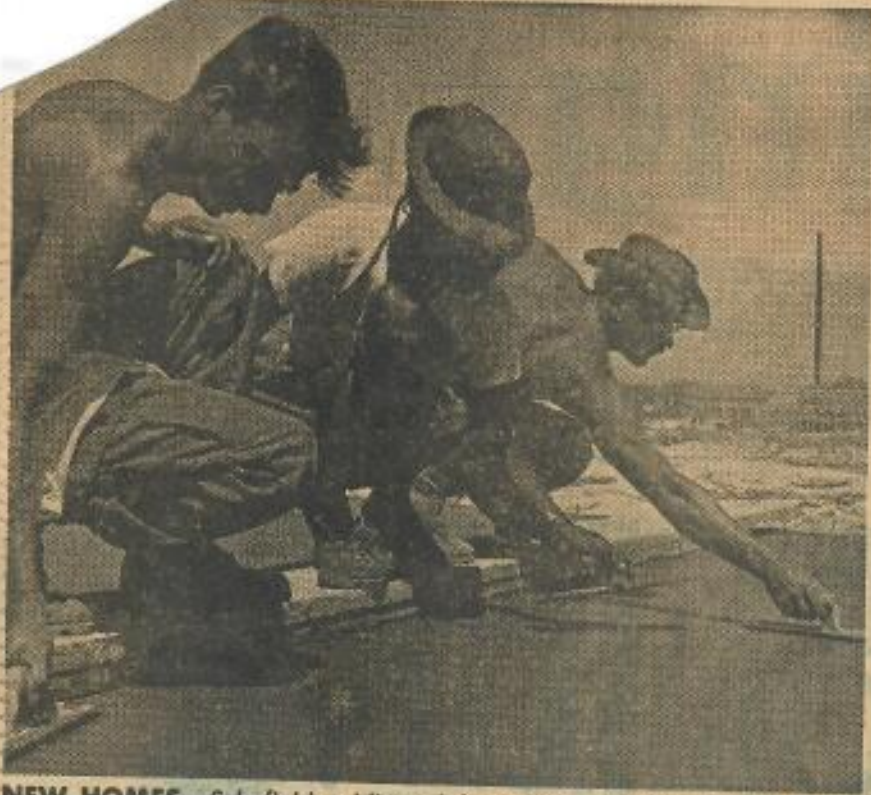
NEW HOMES —Schofield soldiers, left to right, Thomas Turner, Larry Handy and Michael Hollister, pave a floor for a temporary barracks. When the Army finishes its work on Lojwa, the land will revert to a coconut plantation.
