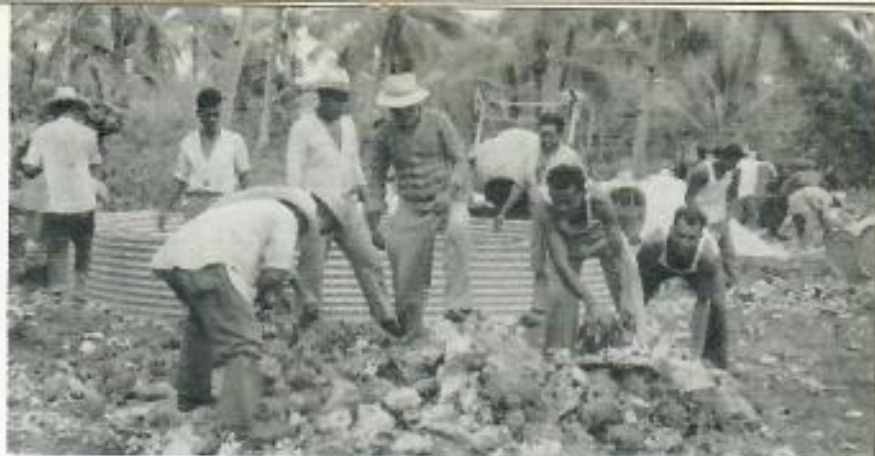
Cooperative working bees are a feature of Niue life: men of a village gather coral for the concrete base of a communal water tank.
