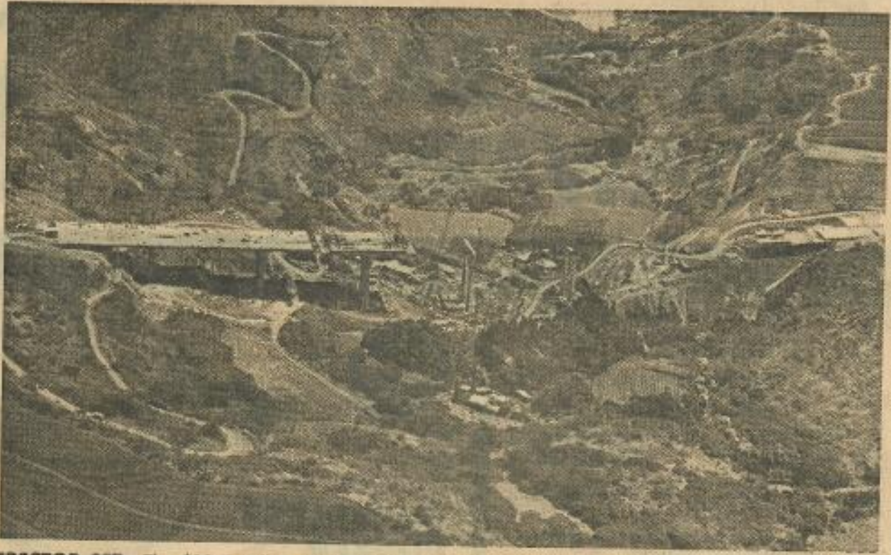
ERECTOR SET —The $13.7 million bridge over Kipapa Gulch between Wahiawa and Mililani Town is expected to be completed in December. The bridge is part of construction that eventually will extend the H-2 Freeway to the North Shore.—Photo by Bob Young.
