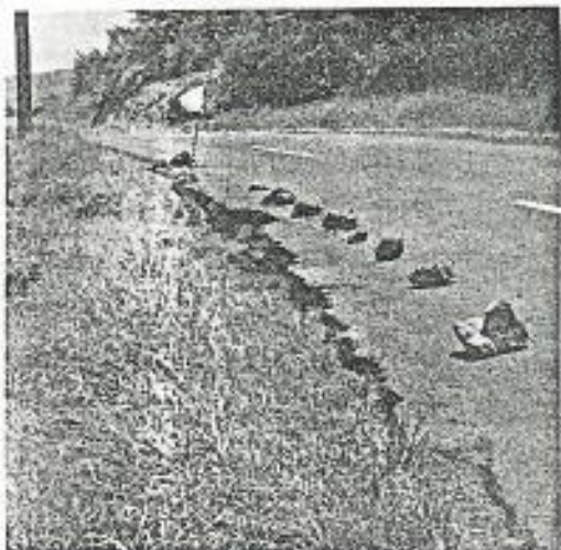
FIG. 9. Crack along roadside south of Kealahou, from the south, showing separation of embankment from edge of pavement due to slumping.
