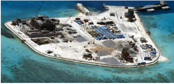
An aerial view of construction at Mabini (Johnson) Reef by China, in the disputed Spratly Islands, in the South China Sea. ((Armed Forces of Philippines))
