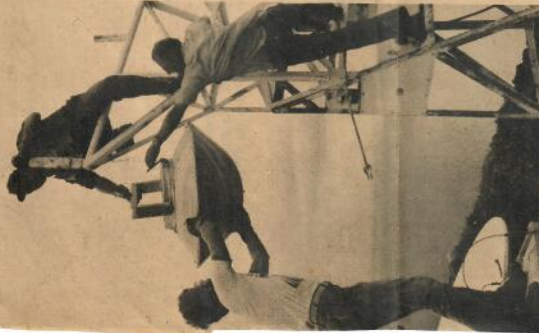
DOWN SHE COMES — Sergeant Robert Goodwin (top) of HMM-262 hands a reflector drum from a Frequency Shift Reflector Radar to Dyna Electronics technicians Jim Miller (left) and Robert Dzina. The dismantling procedure took place atop Lehua Rock, off the coast of Kauai during HMM-262's deployment to Barking Sands. The radar was obsolete and unneeded.
