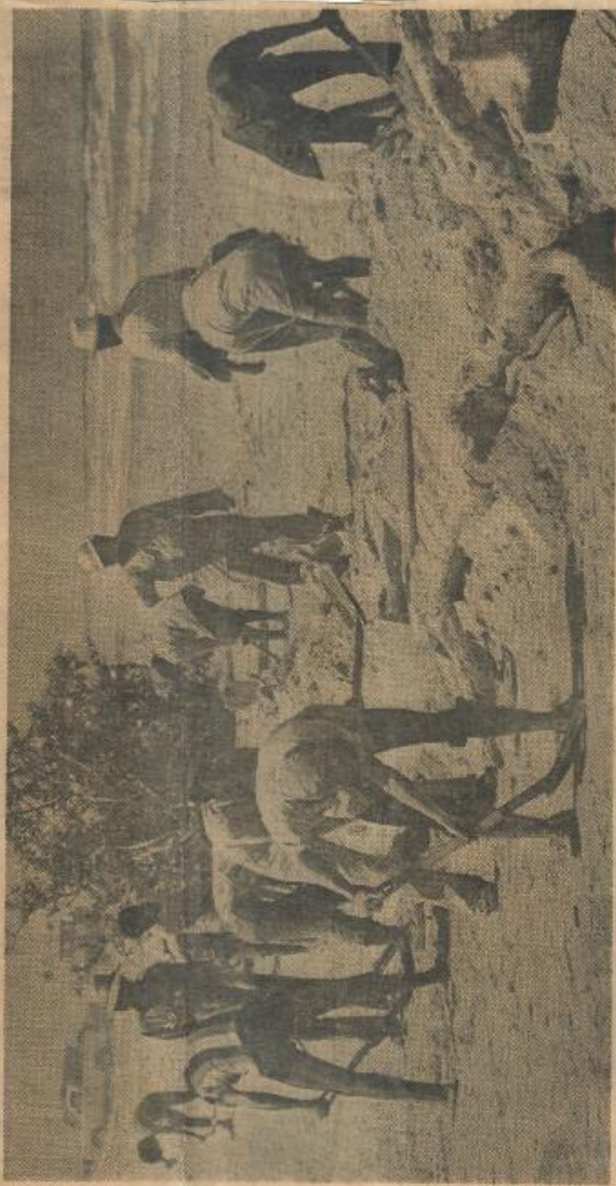
Workers build sand dike on a Mexico beach south of Brownsville, Tex., to protect turtle breeding ground from a growing oil spill. Times photos by Rick Meyer
