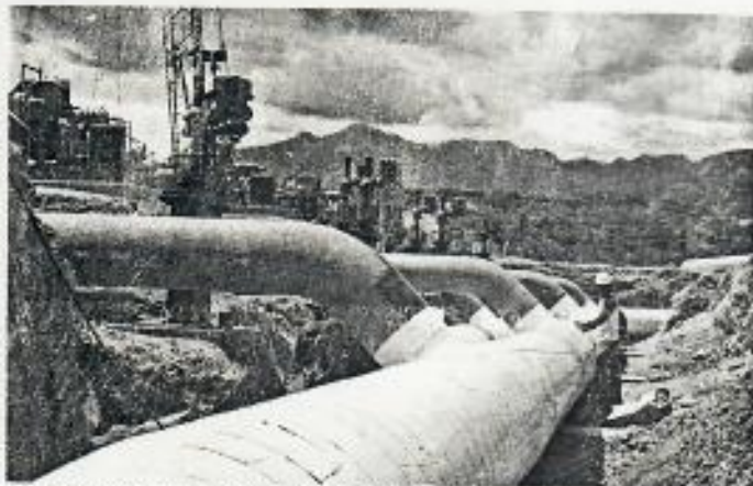
Foothills plant will pump oil 4,000 ft over Continental Divide.
