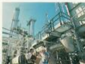
The company's modern synthetic natural gas (SNG) plant at Campbell Industrial park serves the metropolitan Honolulu area.
