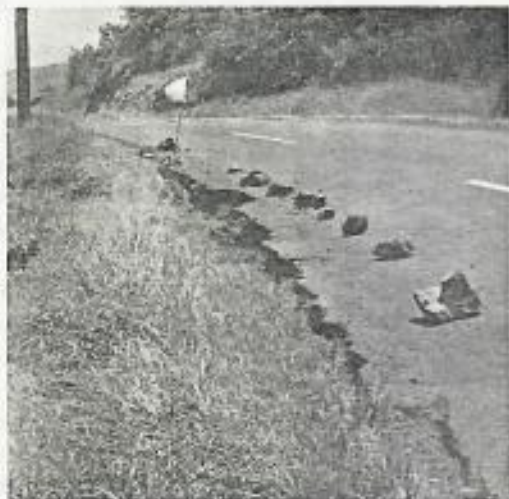
FIG. 9. Crack along roadside south of Kealakekua, from the south, showing separation of embankment from edge of pavement due to slumping.
