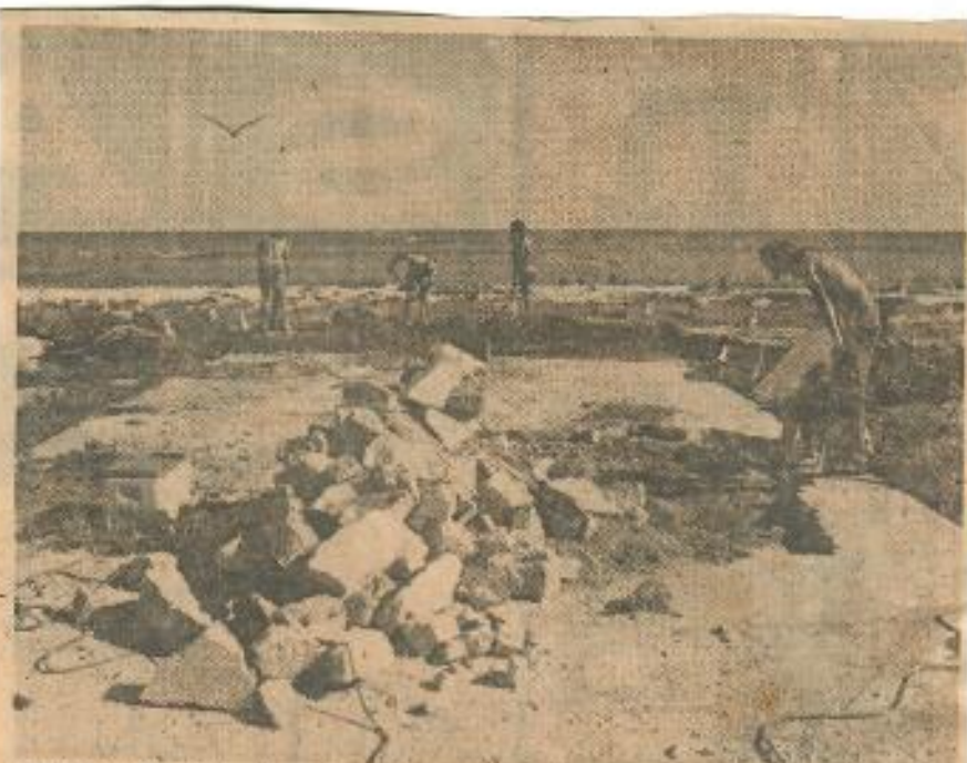
CLEANUP —Scientists break up the principal concrete foundation, measuring 20 by 65 feet, on East Island in order to make more space available for nesting by green sea turtles. —Photo by George H. Balazs.
