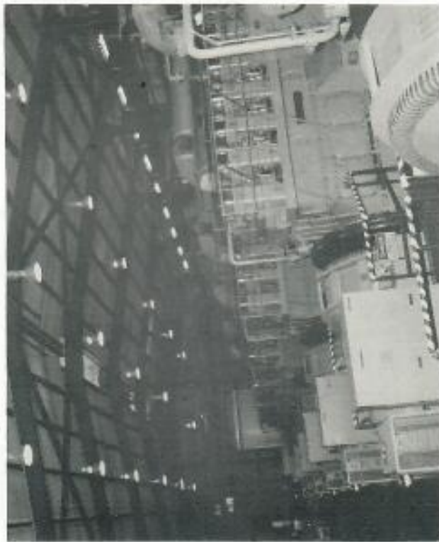
FACILITY NO. 48 - 1,400 KW DIESEL GENERATORS
