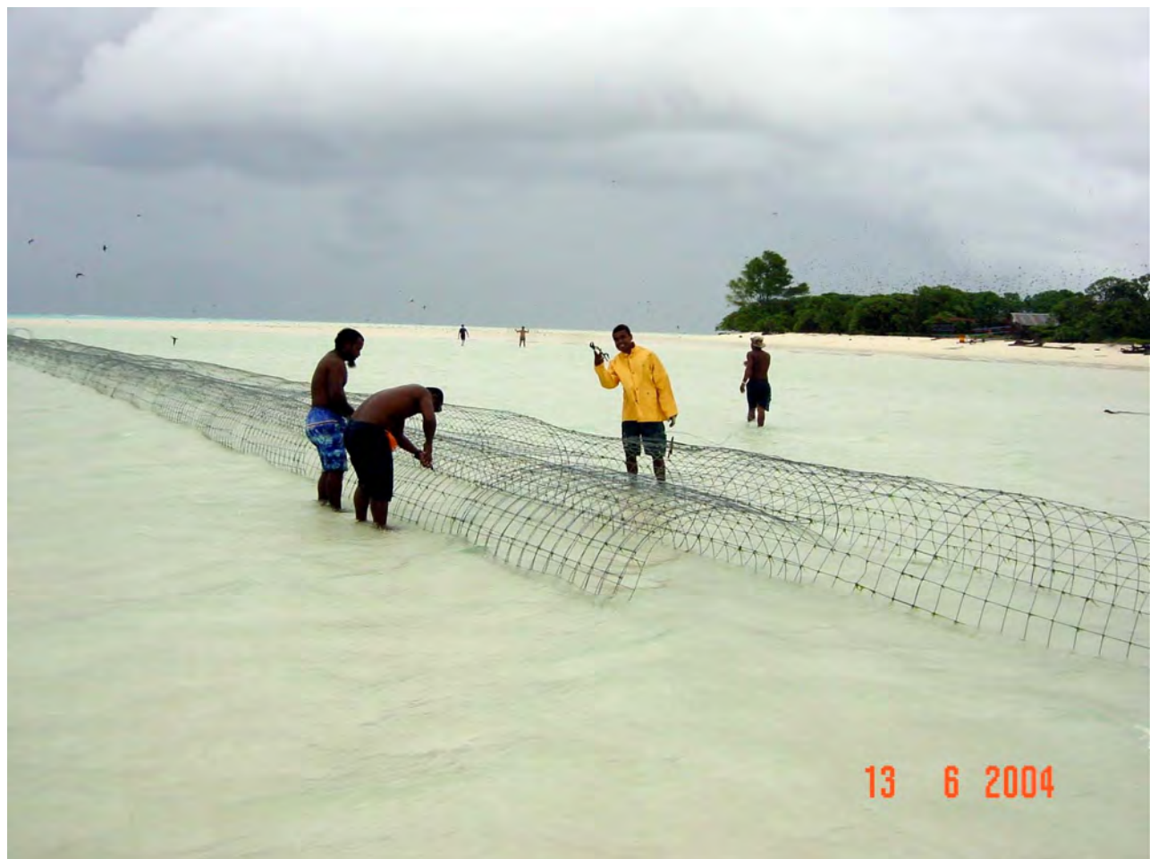
Building a solar powered Biorock reef with Hatahobei young people at low tide to protect Hotsararie from washing away. Notice the huge flocks of sea birds over the island. The dark sky is from a forming Super Typhoon. Photo 2004, Wolf Hilbertz.
