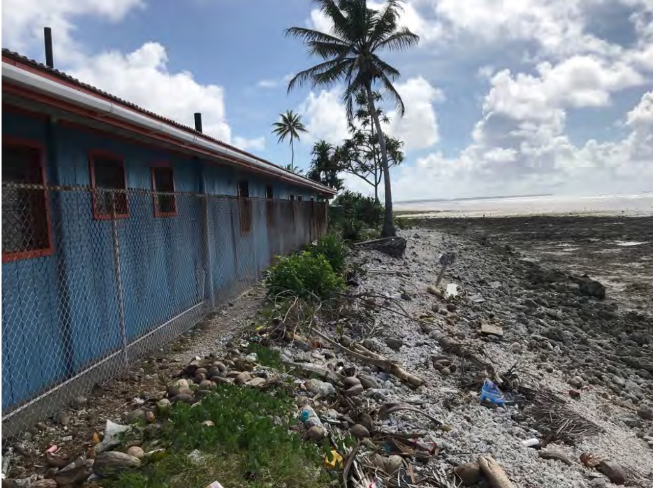
Waves break through the fence and flood the Ejit school during King Tides. 2019 low tide photo by T. Goreau
