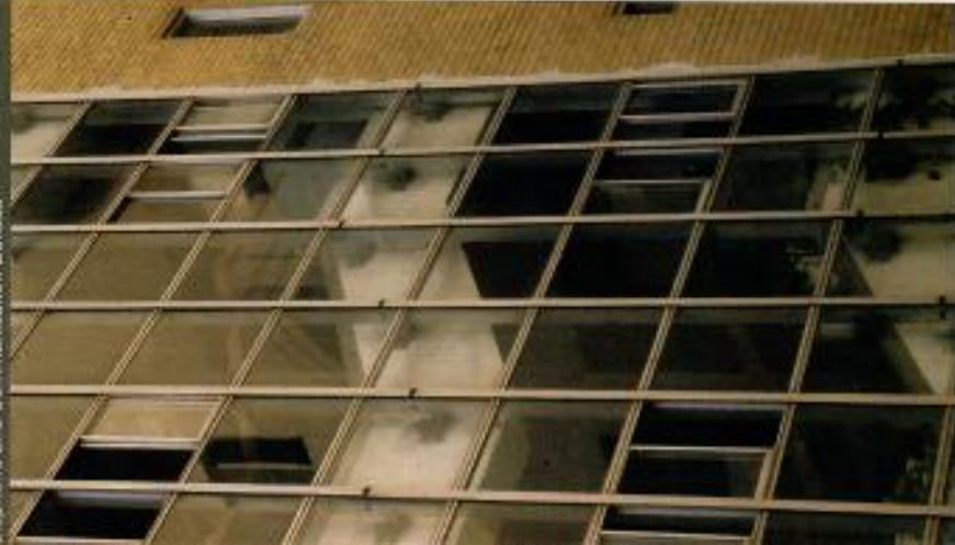
省立成功大學電信局舊營業廳 玻璃窗細節 Detail of Glass Wall of Tainan Telephone and Communication Bureau
