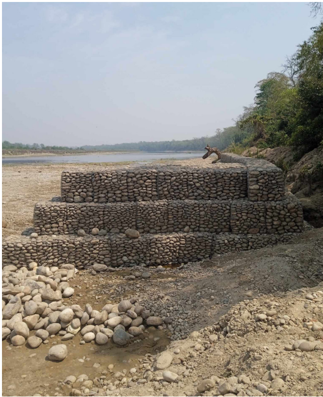
Figure 2. Newly constructed gabion wall along bank of the Rapti River in CNP. Photograph: Bed Khadka.
